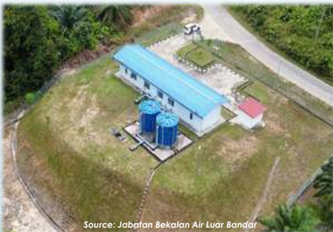
Source: Jabatan Bekalan Air Luar Bandar Sg. Laong Booster Station, Bakong, Miri
